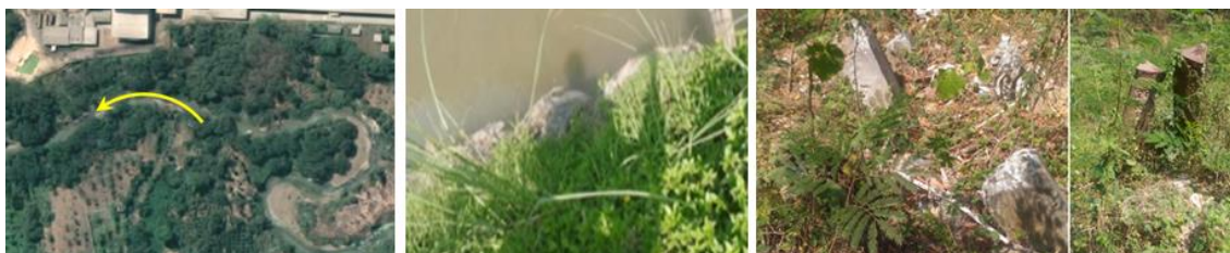
Figure 6. The factory-side river flow (left), streams erode the river slopes on the side of the factory and reduce the retaining power of gabions (middle), and the condition of concrete piles (right)
